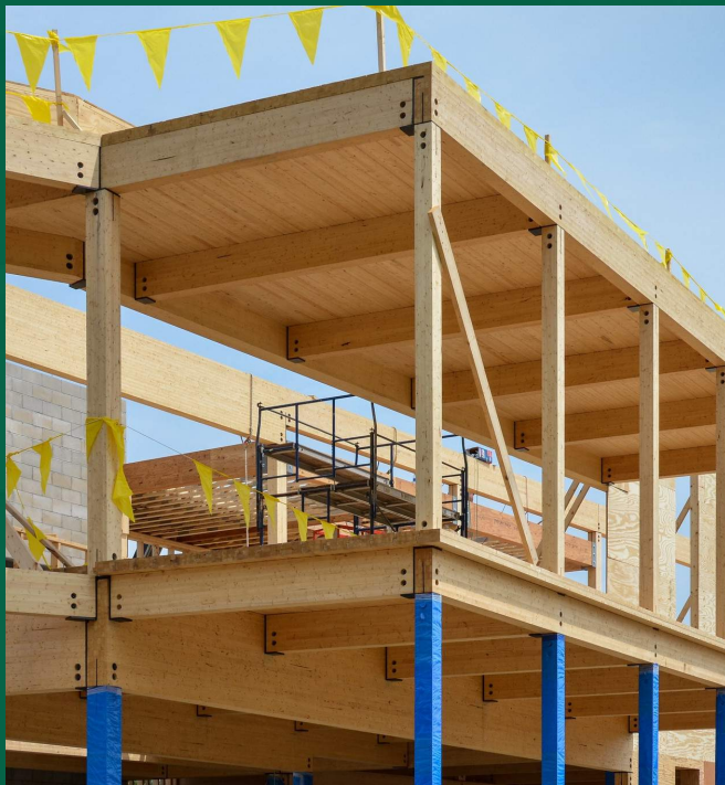
R.W. Kern Center in Hampshire College, Amherst, MA during its construction. The Kern Center is the 17th certified Living Building in the world. Image courtesy of Alexander Schreyer.
