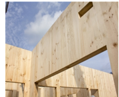
CLT wall elements
