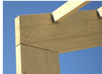
Glulam building frames
